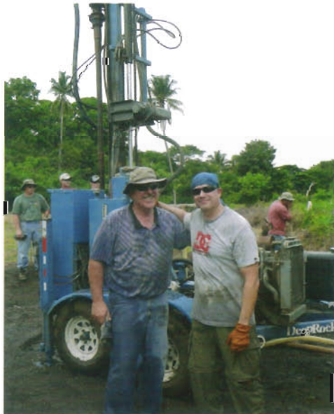
LEFT: Bowman is seen here passing a casement pipe to his team members. TOP RIGHT: Local farmer. BOTTOM RIGHT: John Bowman (left) seen here with friend Mark Gonzales as they catch their breath at a well drill site.
